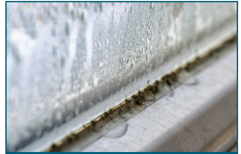
Mold growing on a leaky window sill.
